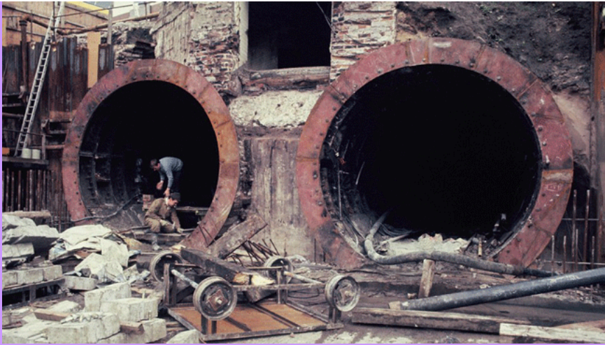
View of tunnels during 1977 reconstruction - the worker on the left shows the small 11' width of each tunnel!
